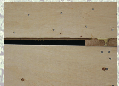
Gap on the side of the box
