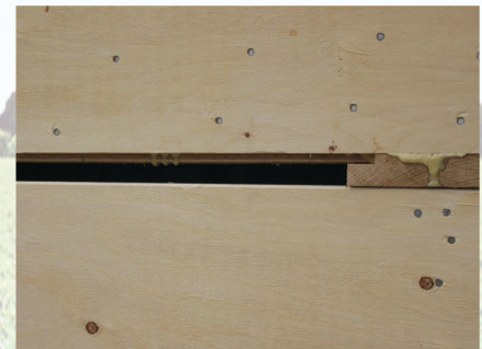
The air can escape through a gap between two boxes.
